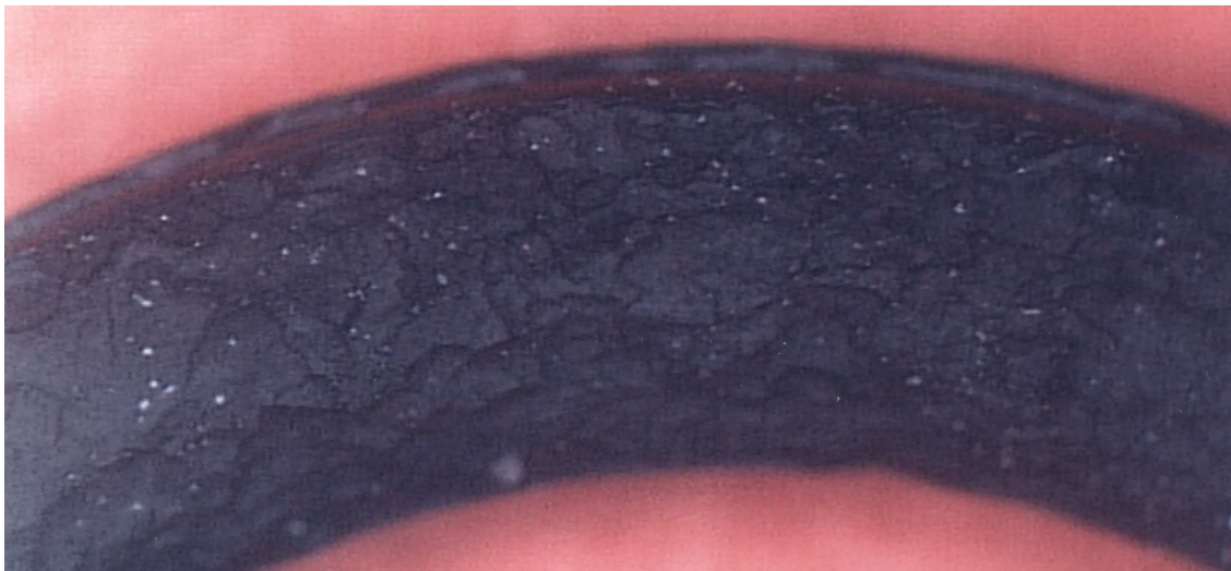
Photo 13: Damage from explosive decompression of air.
